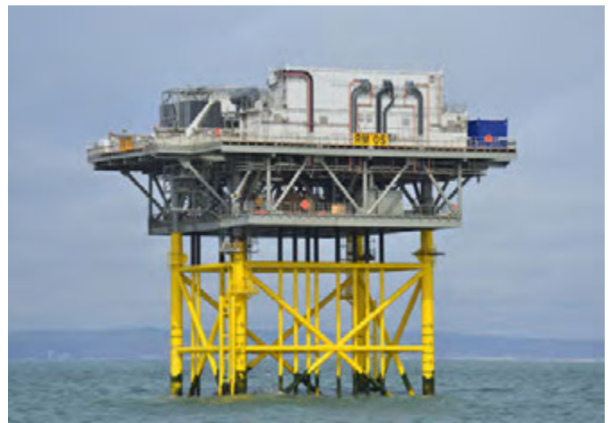
Figure 7: An offshore substation for the operational Galloper Wind Farm
