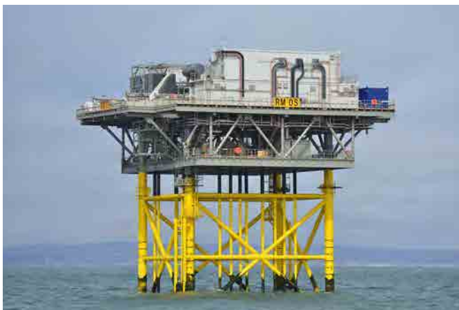
Substation for the Rampion Offshore Wind Farm
