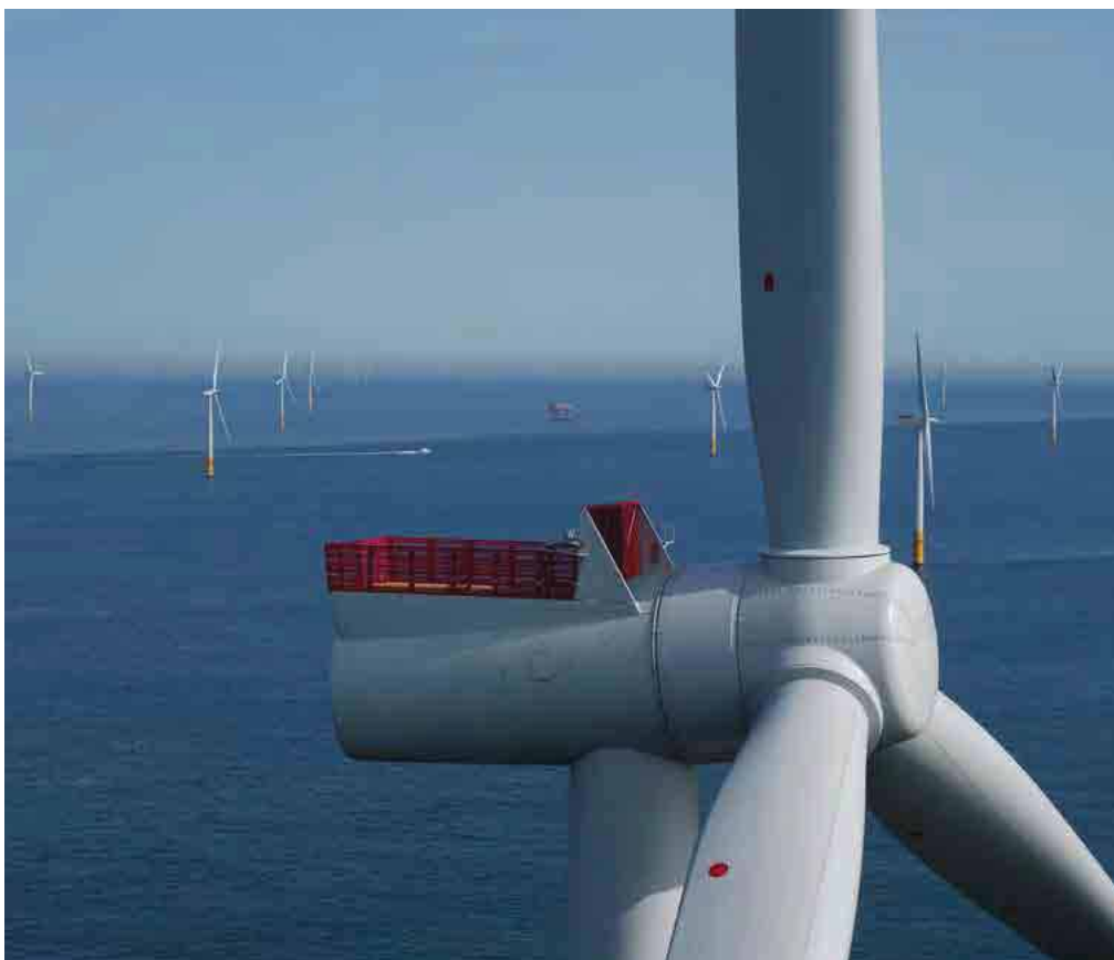
Offshore turbines at the Galloper Wind Farm
